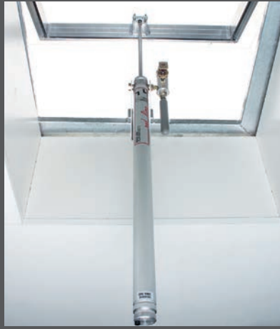
On dome with thermal valve
